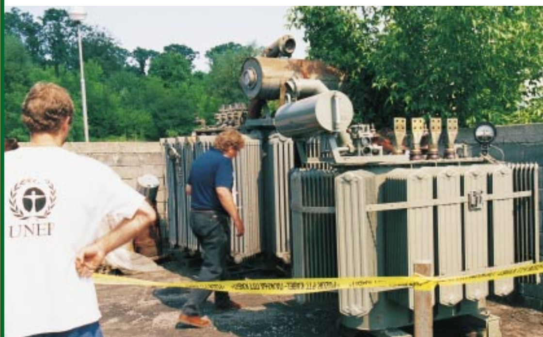
Inspection of damaged transformers
