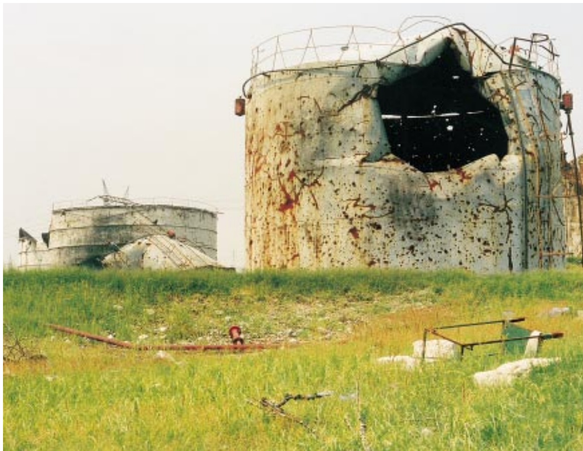
Bombed oil storage facility, Bor
